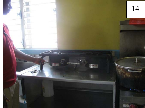
Photo 14 – Stove powered by gas generated from the bio-digester system which is used to prepare meals for the Home. Mr. Whitely demonstrates the process of the gas being generated.
