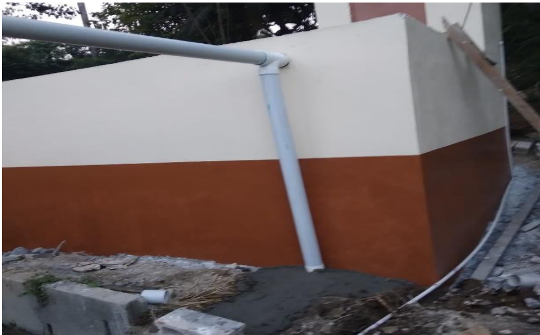
Water Storage tank with conveyance pipes installed
