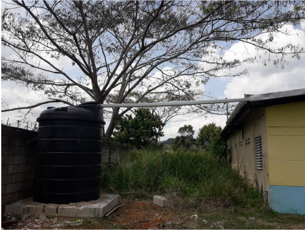
Rainwater harvesting at the Duanvale Community Centre
